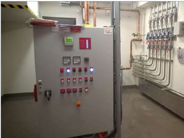
The compact SEM-SAFE® high-pressure water mist unit installed at Lund University.
