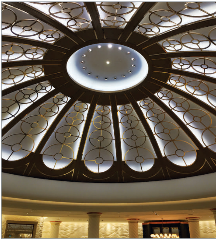
The design of the SEM-SAFE® high-pressure water mist nozzle blends perfectly with the beautiful interior of Ten Trinity Square.
